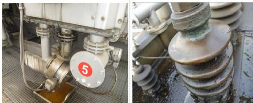
Fig. 1. Oil leakage at the top and bottom of transformer
