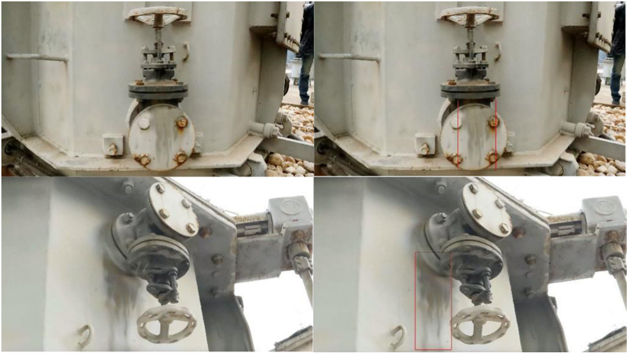
Fig. 8. Comparison of the detected oil leakage
